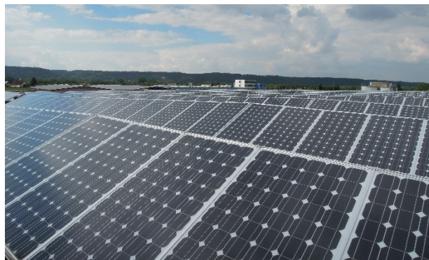
187 kW-Anlage Petersen-Allpa in Aitrach
